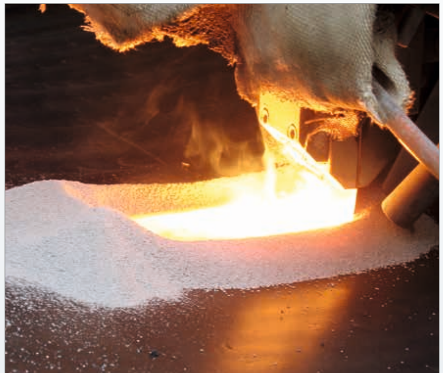
Right: ESW cladding of an Inconel 625 protective layer onto a SA 516 Gr. 70 vessel for the desalination industry. Welding parameters: 1050-1180A, 24-25V, 19.8-21.9cm/min. Strip dimensions OK Band NiCrMo3: 60 x 0.5mm.
